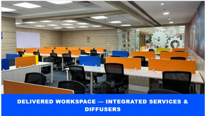
Logix Cyber Park Tower D • Linear AC Diffusers & Troffers • Coordinated Ceiling Integration
